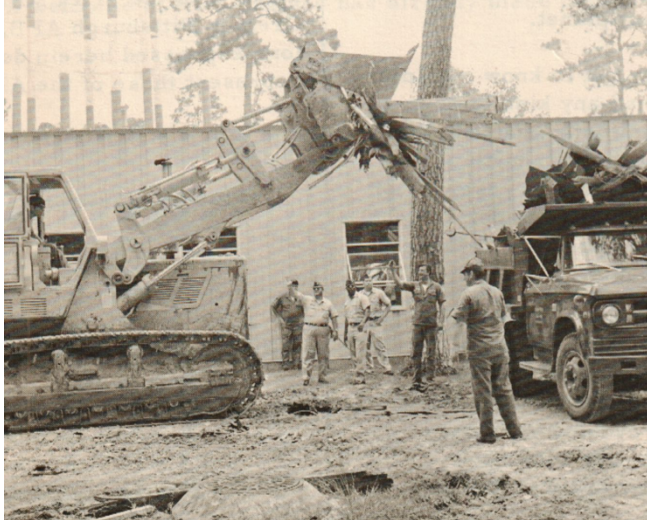
901 CEF complete demolition of buildings dating from World War II at Keesler AFB, MS. (USAF photo)
